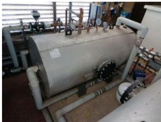
Example of Calorifier 2
