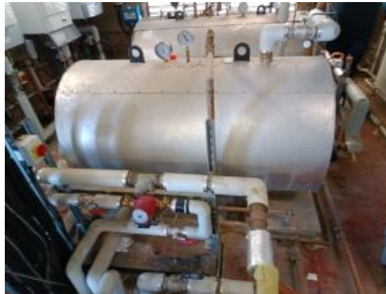
Example of Calorifier Cylinder 1
