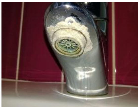
Example of scale present on tap outlet and aerator.
