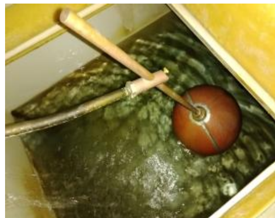
Example of Cold Water Storage Tank 1 internal view
