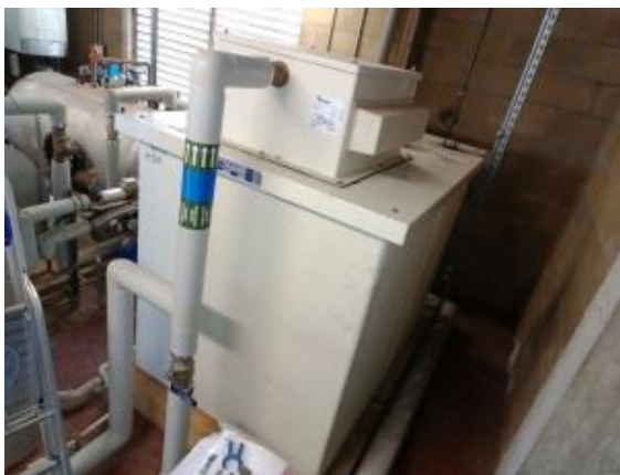
Example of Cold Water Storage Tank 1
