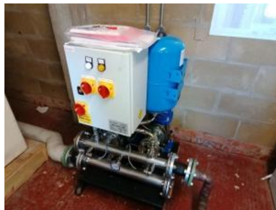
Example of twin pumps associated with Cold Water Storage Tank 1
