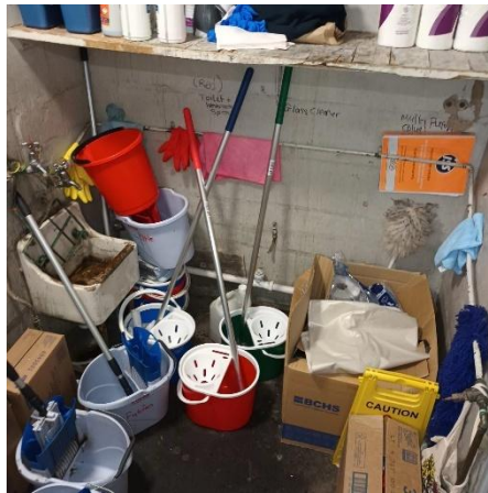
Photo 7 - view of seized cold-tap located in 2 nd floor cleaners which has been identified as a blind end.
