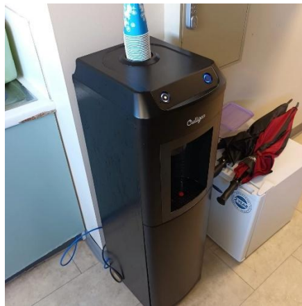
Photo 8 - view of typical water cooler found throughout the medical centre
